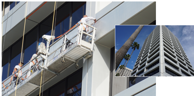
Newport Center, Newport Beach, CA, metal surface prep (left) and completed (right)
