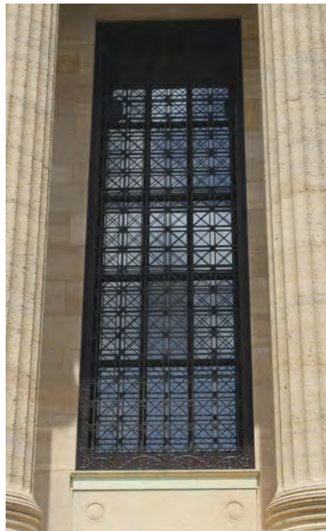
The scale, intricacy, durability, and high level of craftsmanship of the bronze window grilles at the Philadelphia Museum of Art are an important and beautiful part of the building’s aesthetics. Photo courtesy of PMA.
