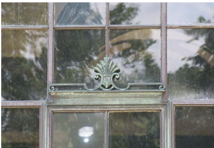
A close-up of the bronze window ornamentation at the Rodin Museum shows how badly weathered it was prior to restoration. Photo courtesy of the Rodin Museum.
