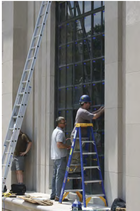
Workers reinstall the bronze windows at the Rodin Museum following cleaning and repatination. Photo courtesy of the Rodin Museum.
